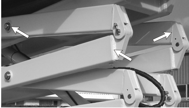
Figure 7.19 - Structural Damage and Welds
