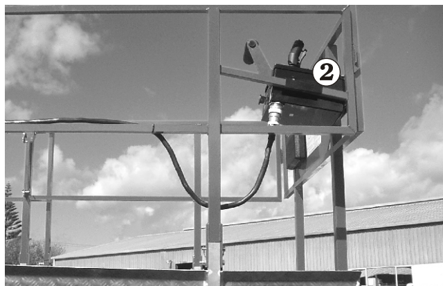
Figure 6.1.2 - Control Box Location, Platform Position
