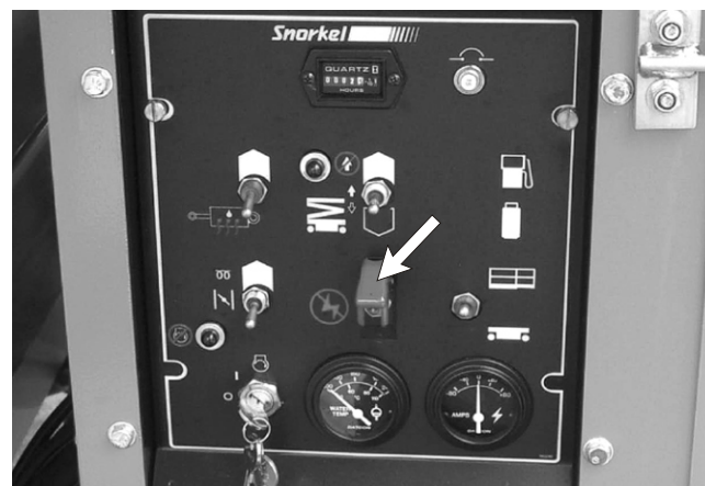
Figure 8.1 - Emergency Stop Switch at Ground Control Box
